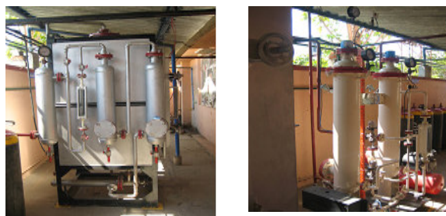
Fig4,5. Ammonia Cracker and Dryer.
