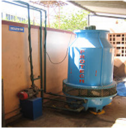
Fig6. FRP water cooler tower.
